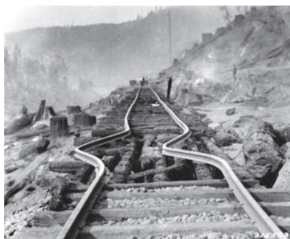
Figure: 2.1 (above) Gap between rail lines. (below) Crooked lines because of hot weather
